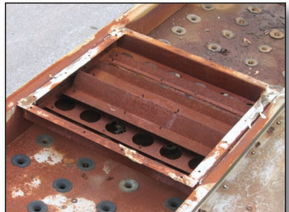
Corroded Hot Water Basin
